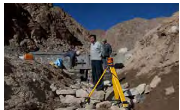
Chewang Norphel watches over construction of a shallow pool, which will hold an artificial glacier in the Ladakh region of north India. Photo: Ecofriend.com
